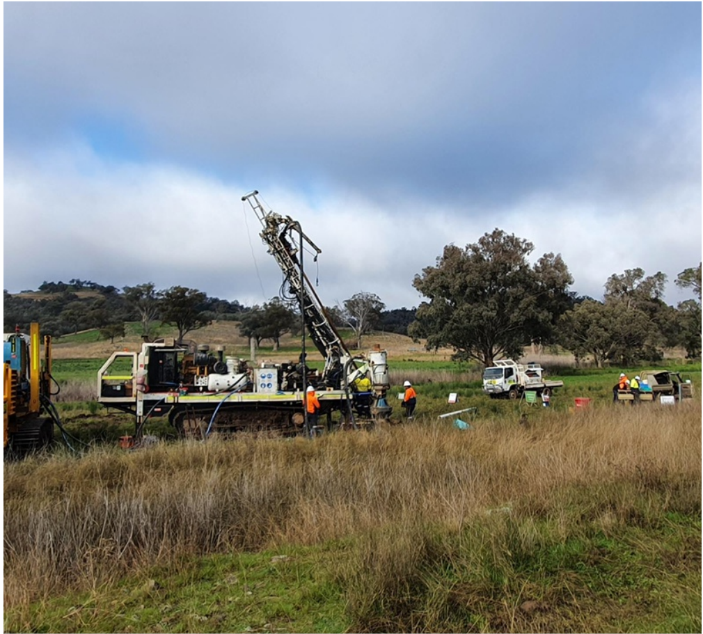
Track mounted Sandvik UDR650 multipurpose drill rig has arrived on site to expedite the Phase 1 resource drilling.
